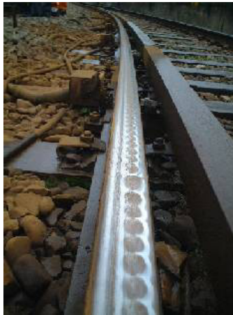
Figure 1: Example of rail corrugation.
